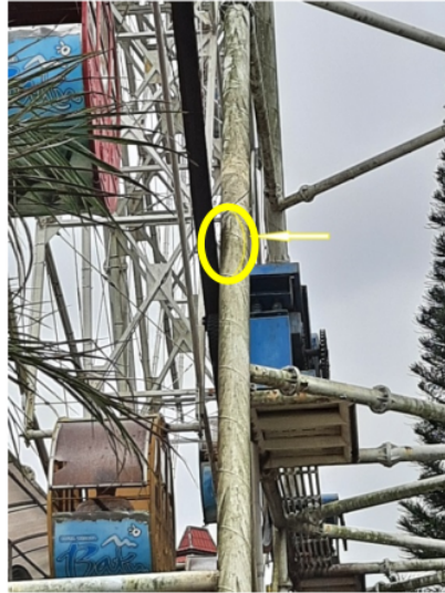
Fig. 4. Friction between the rim and the support pipe that causes happening scratches/flaws
