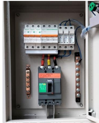
Gambar 2.1 Panel Kontrol 3 Phase
