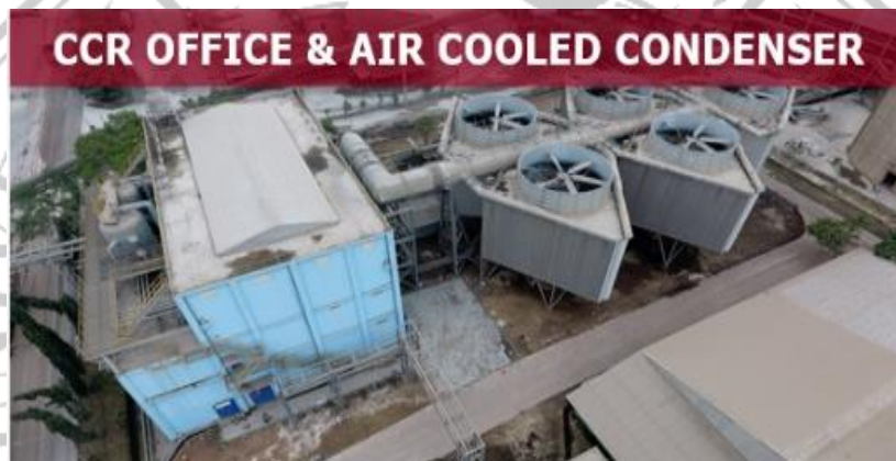
Gambar 2.2 Air Cooled Condenser
