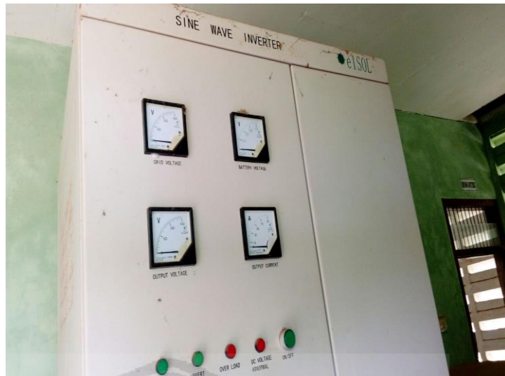
Gambar 3.5 Inverter PLTS kalipucang
