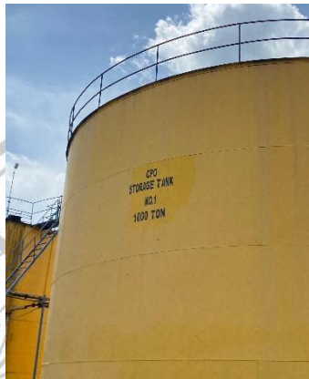
Gambar 14. Storage tank No.1
