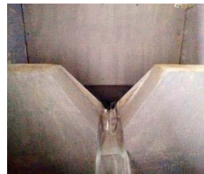
triangle threshold downstream of the weir
