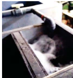
initial water storage tank (wst)
